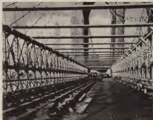
The new steel grid deck begins to take shape on the main span.
